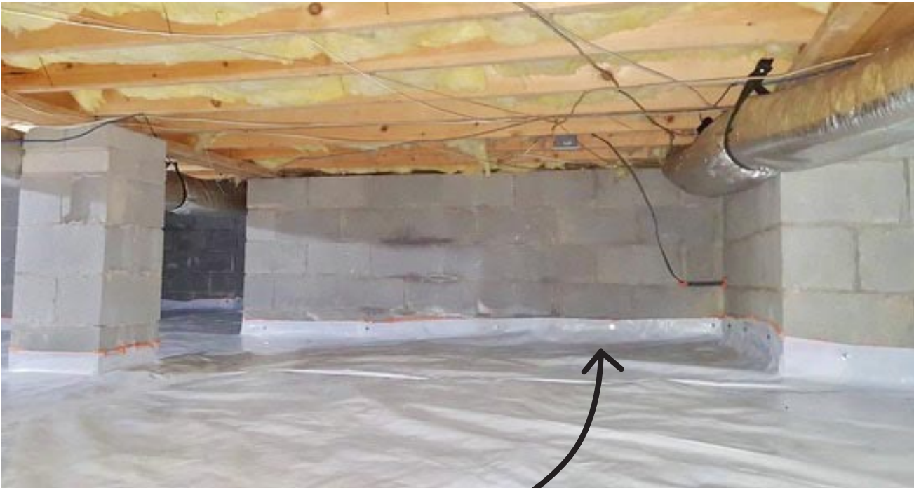
Complete crawlspace, ducts lifted, heavy duty vapor barrier laid down, nailed and adhered throughout crawlspace
