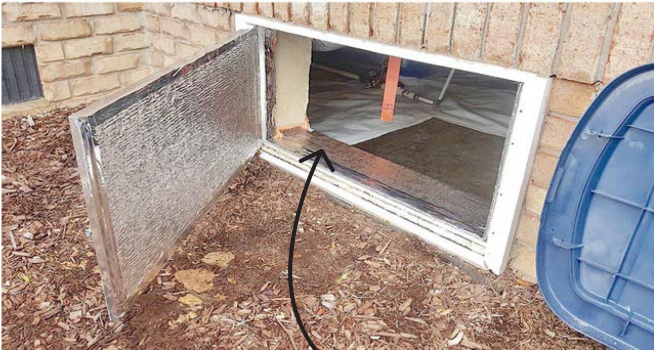
Door Gasket, door insulation, and door entry padding complete. Nobody seals it better than SHS!
