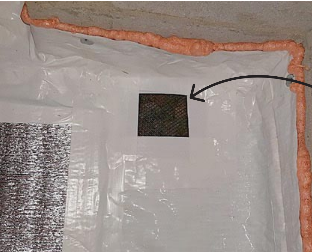
Crawlspace built since 1993 should have a "LOW-POINT-DRAIN"
