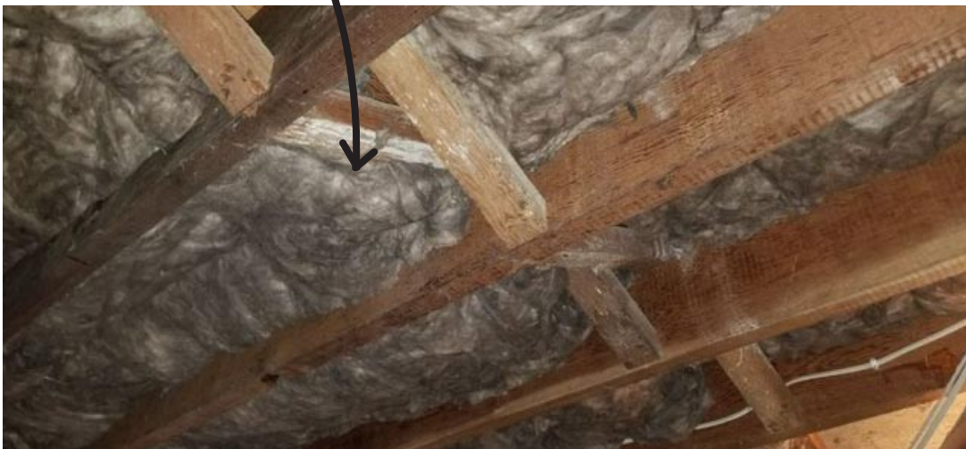
When adding new insulation we use EcoBatt, R-19 Insulation which is formaldehyde free
